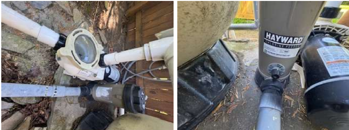
Pentair Superflo 1 HP Pump and Haywared Inline Chlorinator
